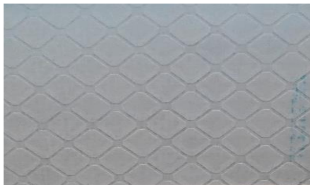
Fig. 5. Asbestos ceiling board
