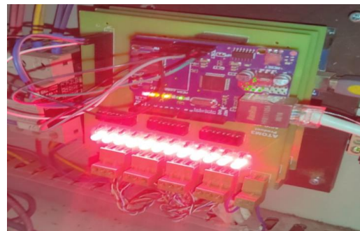
Fig. 4. Hardware installed at Site
